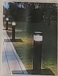
④ Bollard Lights
