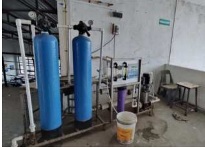
R O Plant
